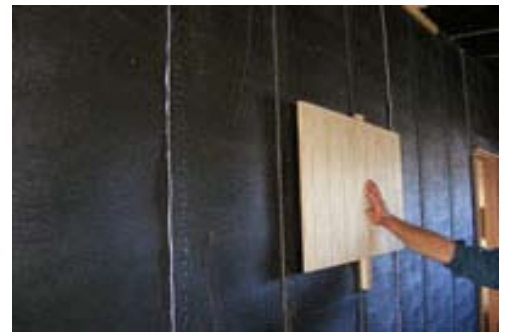
Hidden behind wall panelling (inset), the Wavebar shuts in power-tool noise from escaping a new purpose-built hobby shed)
